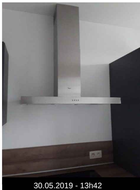
Photo 17 (Cuisine / Hotte aspirante / Neuve)
